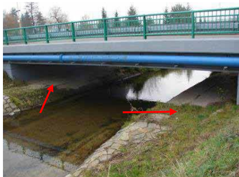
Figure 37 An example of the surface under the bridge with the dry passage for mammals and other terrestrial animals
