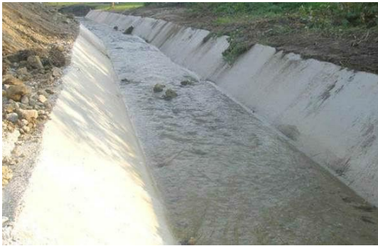
Figure 39 Example of undesirable solution of watercourse regulation
