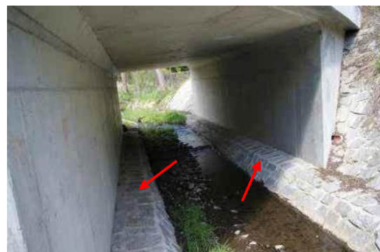
Figure 38 Photograph as an example of box culvert with the dry part of the passage for mammals and other terrestrial animals
