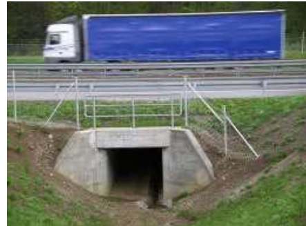
Figure 32 Photograph as an example of adjusted box culvert below the road level, for small terrestrial animals
